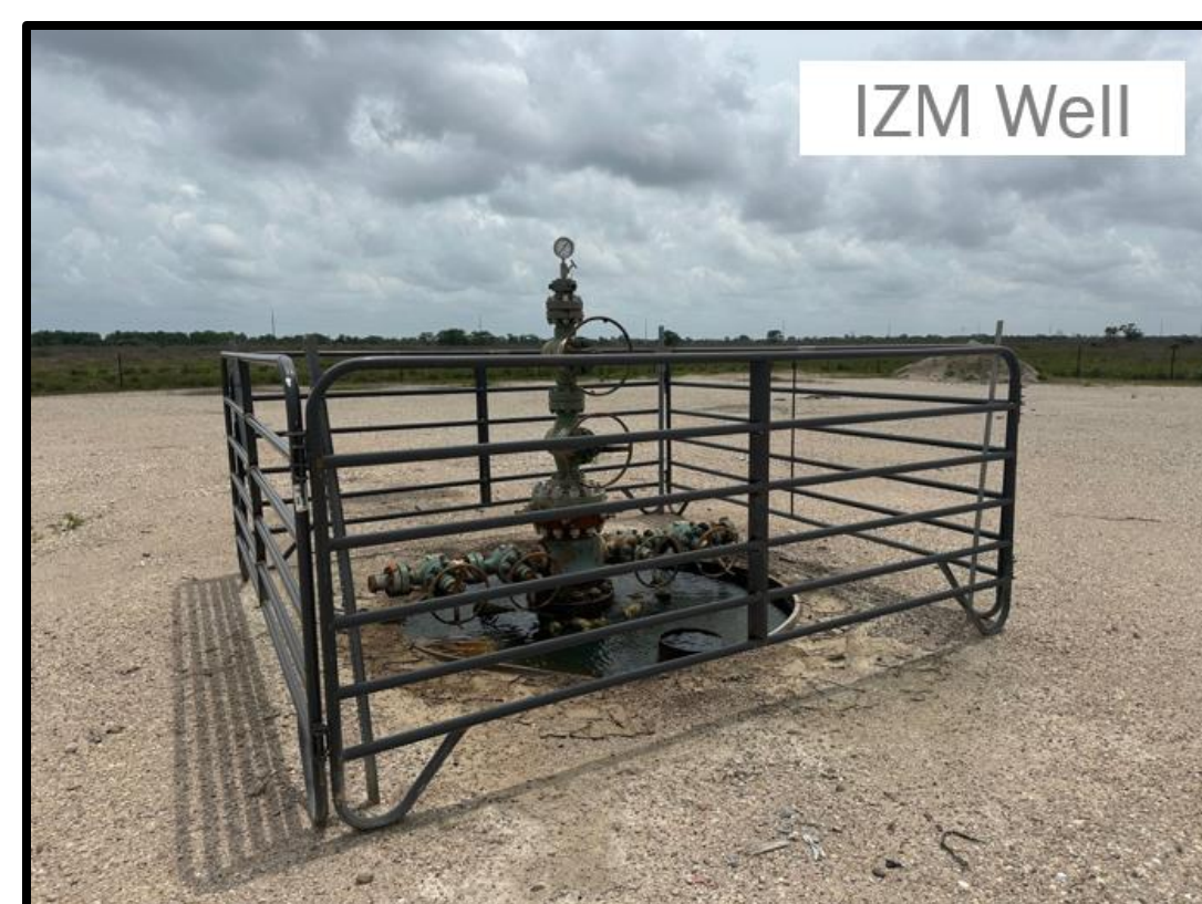
In-Zone Monitoring Well: Illustrating the size and footprint of a well head.
